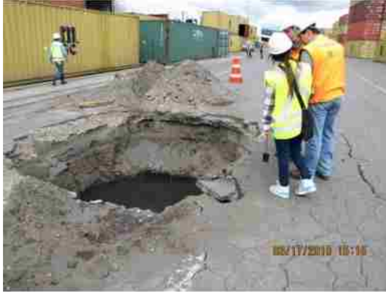
Figure 6-7: Sink Hole at the Port of Coronel (GEER 2010)
